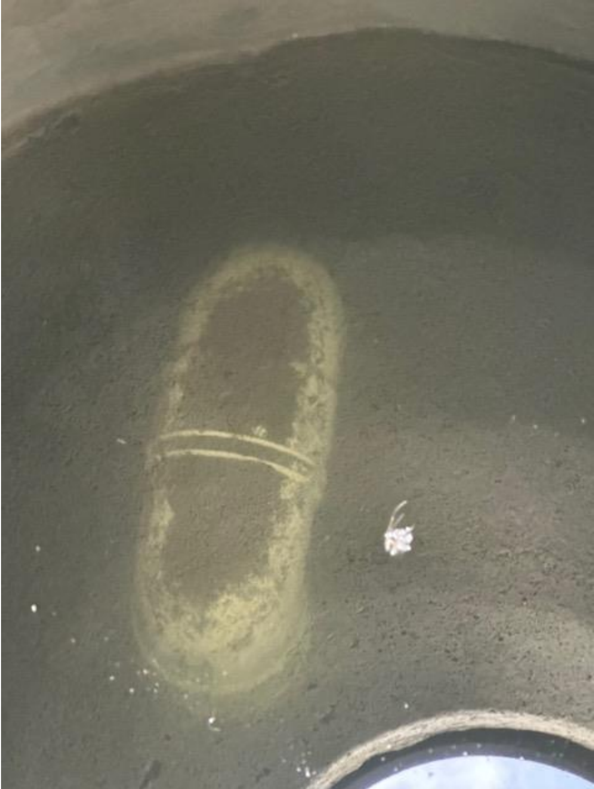
Overflow Structure Inside Montage Drywell Manhole
