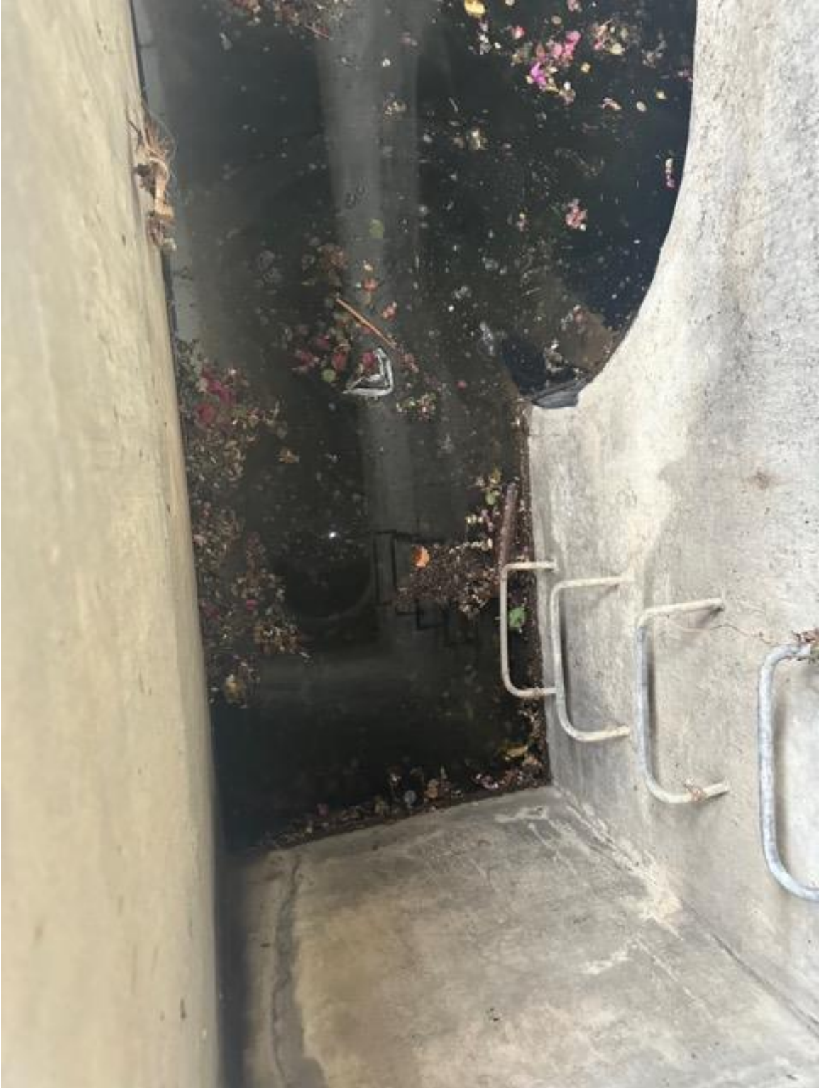
Inside East Stormwater Box Culvert and Connecting Drywell Inlet Pipe and Access Ladder
