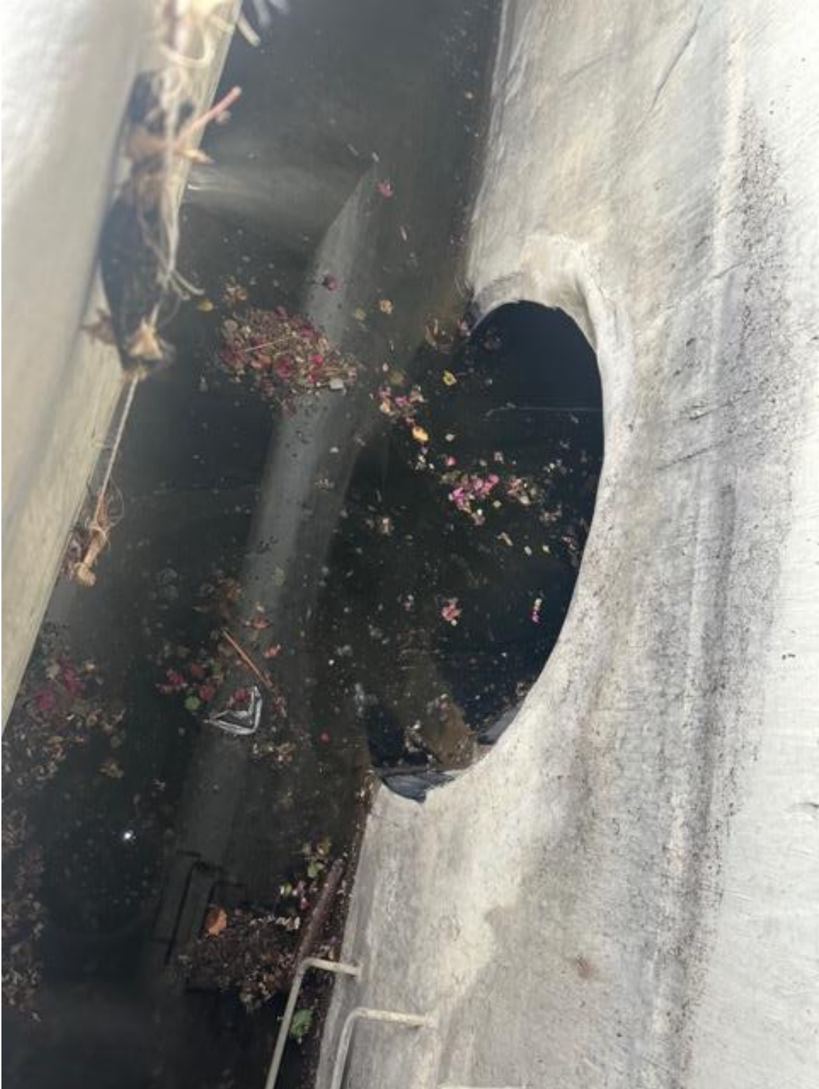
Inside East Stormwater Box Culvert and Connecting Drywell Inlet Pipe and Access Ladder. Mosquito Mitigation Package Hanging from Culvert Grate
