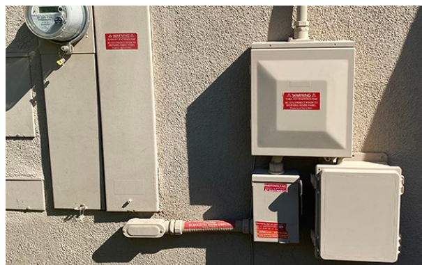
CORRECT: Boxes and conduit are painted
