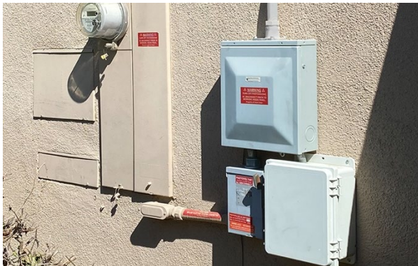
INCORRECT: Boxes and conduit are not painted
